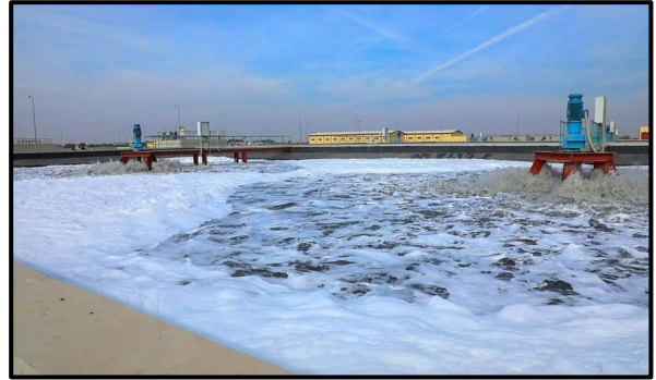
Mixers Works at the Precipitation Basins-Al-Hai Central Sewage Treatment Plant© Al-Hai District Sewers Directorate
