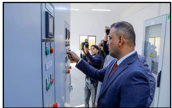
Wasit Governor launches the Operational Works at Al-Hai Central Sewage Treatment Plant© Al-Hai District Sewers Directorate
