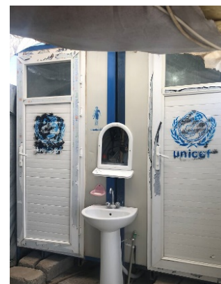
WASH Facilities, Bersive IDP Camp, Duhok. (Credit: OCHA, H. Stauffer)
