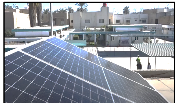
Solar panels on top of a school constructed by UNICEF in Basra © UNICEF
